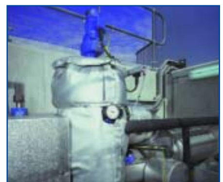
Bollfilter 6.18 filter installed upstream on the waste water supply.
