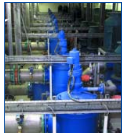
The Bollfilter Pre Screening installation.
