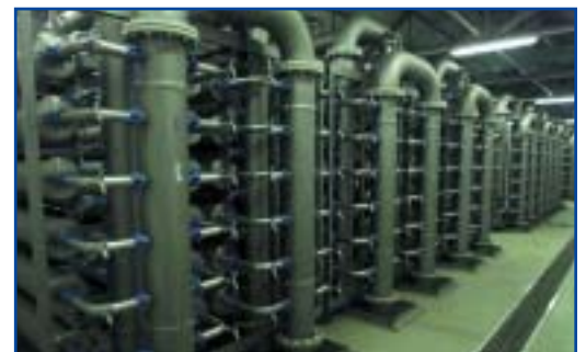
The Keldgate Ultra Filtration Membrane Plant.
