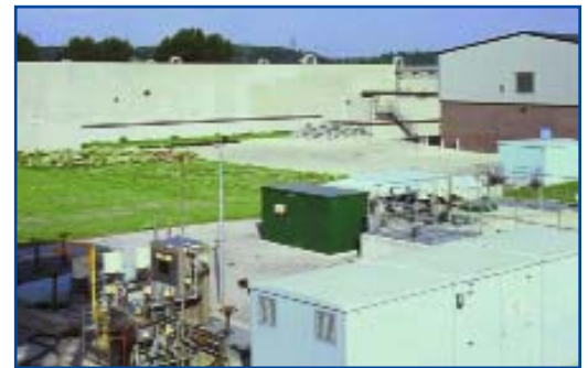
The Secondary Treatment Plant at Wessex Water's Avonmouth site.
