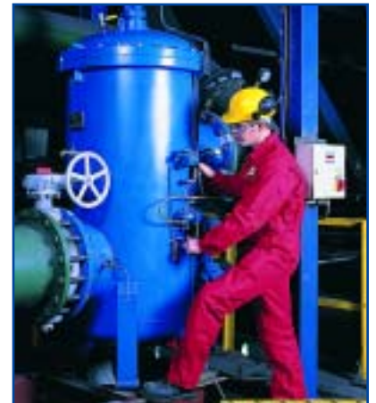
Bollfilter Field Engineer, Paul Moore, carrying out routine maintenance.
