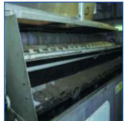
Sludge thickening belts are cleaned using filtered waste water (guard removed for photograph).
