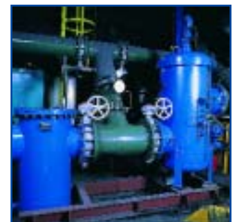
Bollfilter 6.18 filter installation.
