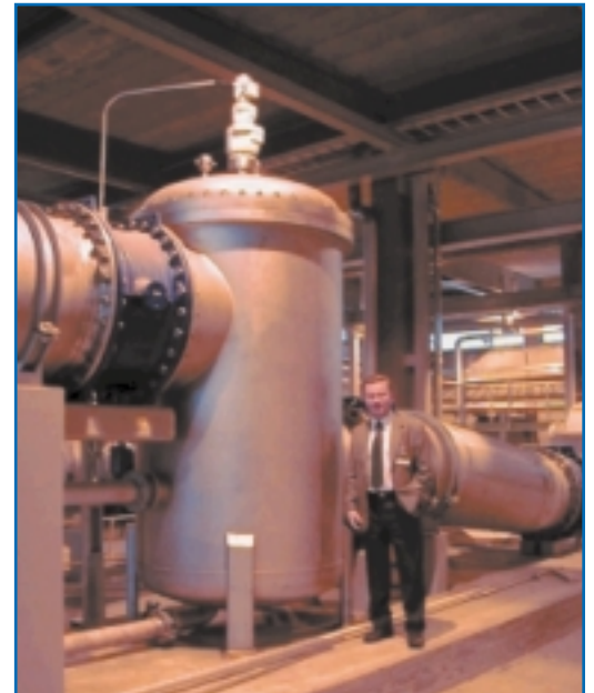
Bollfilter system installed at UPM-Kymmene Oyj, Tervasaari..
