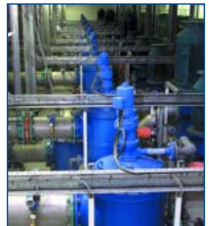
The Bollfilter Pre Screening installation.
