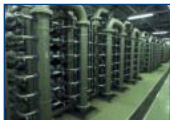
ABOVE. The new plant, which features four banks of primary membranes.
