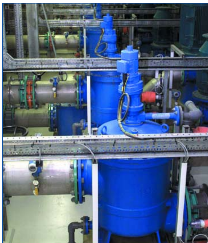
ABOVE. The Bollfilter installation comprises eleven 6.19 automatic filters.
